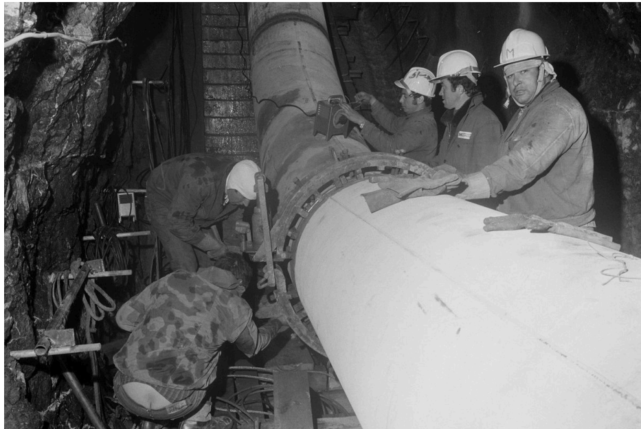
CONSTRUCTION OF A NATURAL GAS PIPELINE IN MEIRINGEN; BRIENZER ROTHORN TUNNEL, SWITZERLAND
