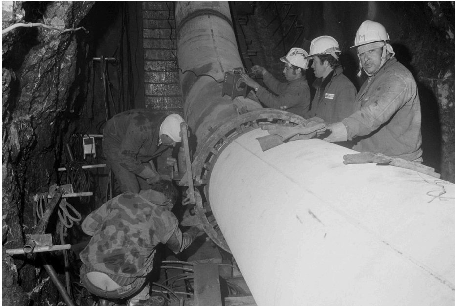
CONSTRUCTION OF A NATURAL GAS PIPELINE IN MEIRINGEN; BRIENZER ROTHORN TUNNEL, SWITZERLAND
