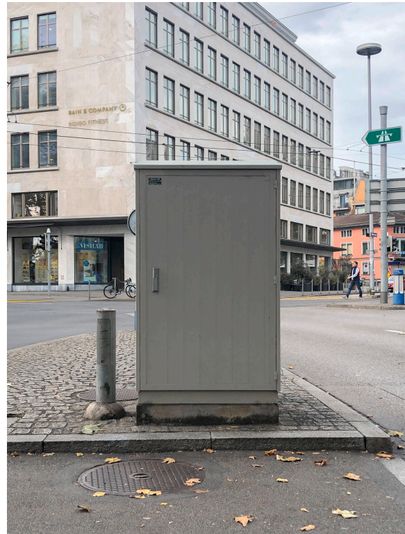
ELECTRICITY BOX Connecting city and country
