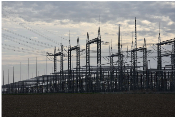
DIFFERENT TECHNICAL ELEMENTS OF ELECTRICAL SUBSTATION OBERZIER
