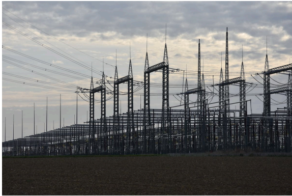
DIFFERENT TECHNICAL ELEMENTS OF ELECTRICAL SUBSTATION OBERZIER
