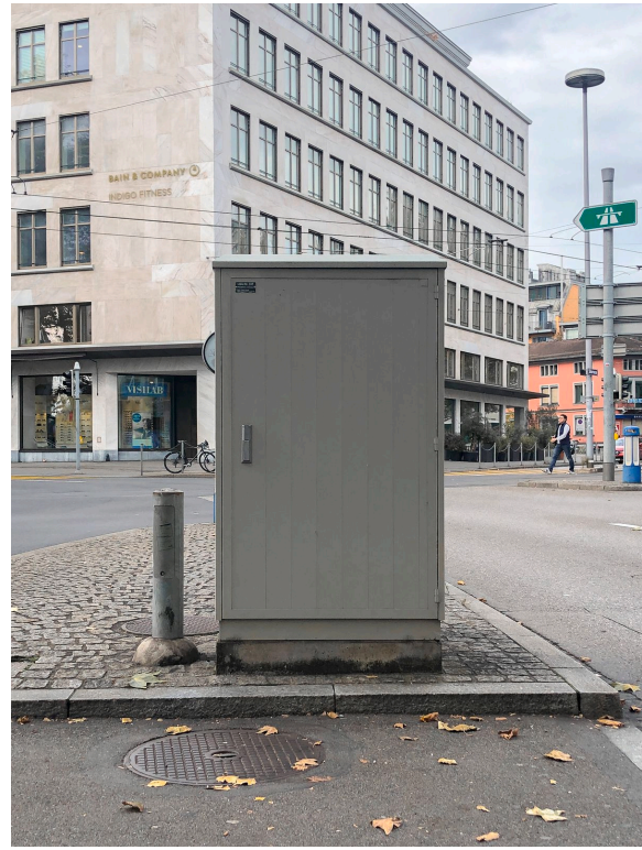
ELECTRICITY BOX Connecting city and country
