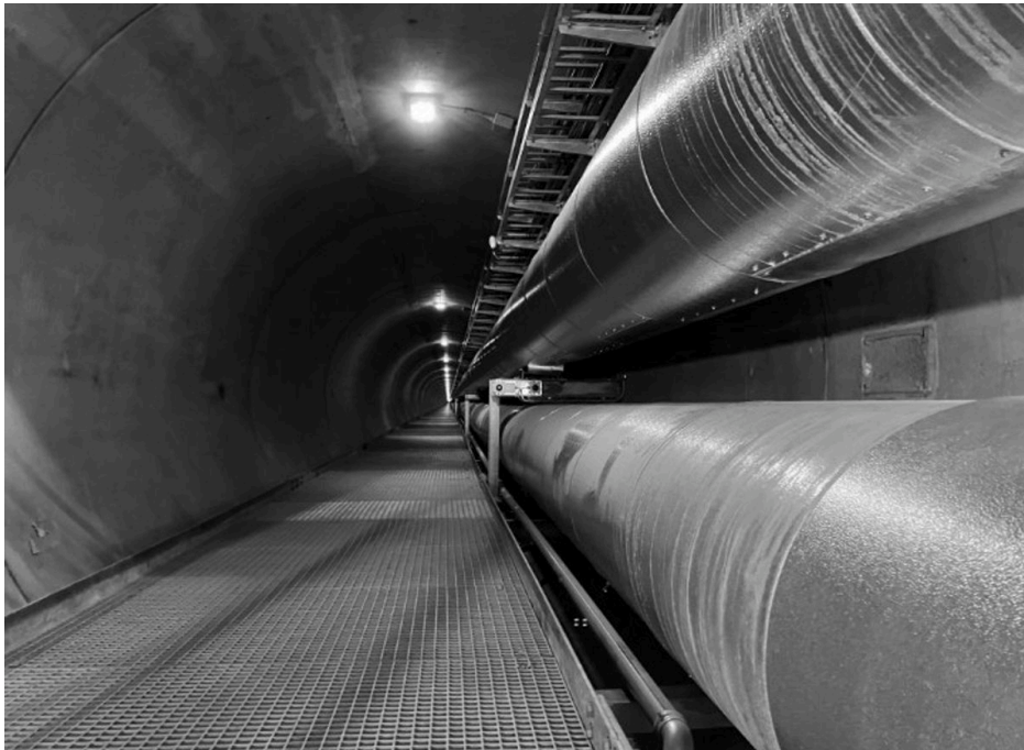
District heating pipes. Source: Baublatt, 2022.
