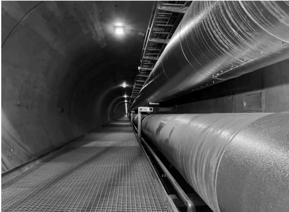
District heating pipes. Source: Baublatt, 2022.
