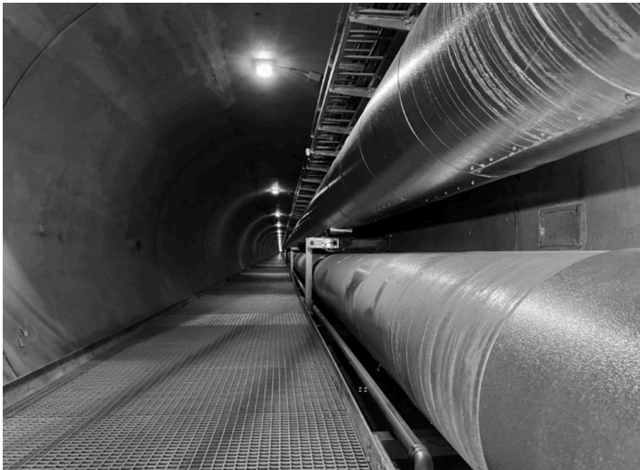
District heating pipes. Source: Baublatt, 2022.
