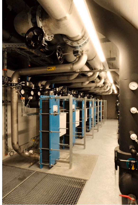
Water-to-water heat exchanger. Photograph: the authors, 2025.
