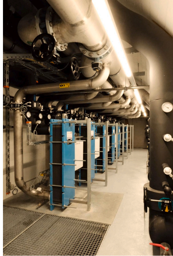
Water-to-water heat exchanger. Photograph: the authors, 2025.
