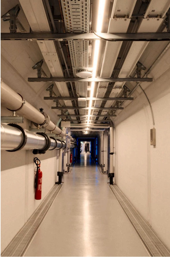
Hallway to the server rooms
