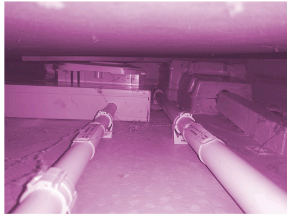
OPTIC FIBRE SERVICE ENTRANCE
