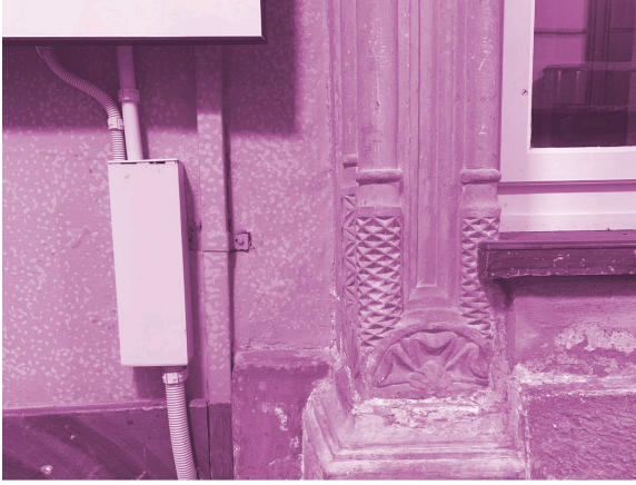
OPTIC FIBRE SERVICE ENTRANCE
