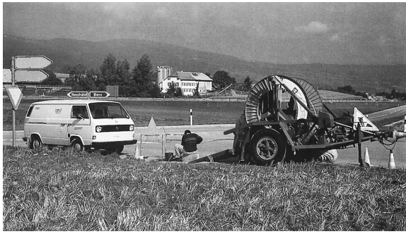
Laying of Fibre Optic Cables Between Zurich and Bern. Source: J.-F. Zürcher, 1986.
