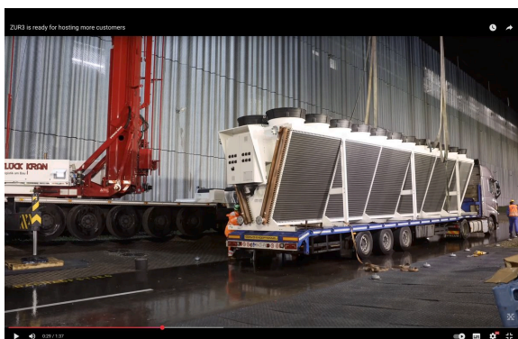
Transport of the chillers for installation on the roof. Screenshot from YouTube video by DigitalRealty Switzerland, 2024.
