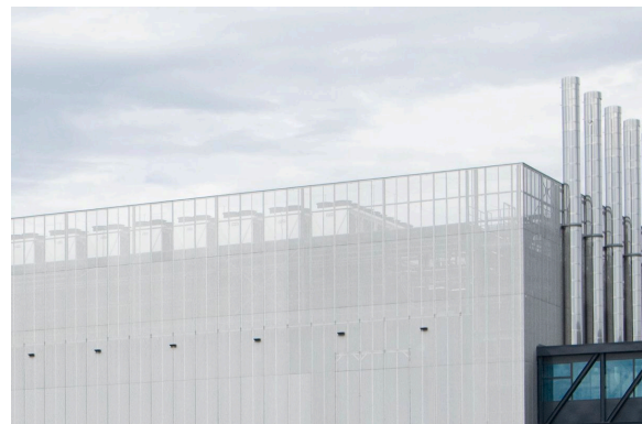
Cooling Infrastructure on the roof of the data center ZUR3, DigitalRealty Glattbrugg. Photograph: AOT, 2025.
