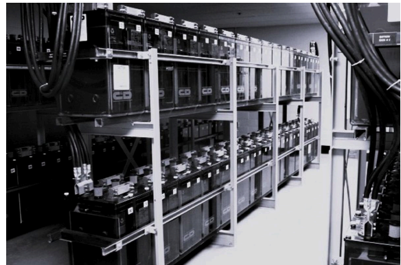
UPS batteries. Source: Kim Otte, 2010.
