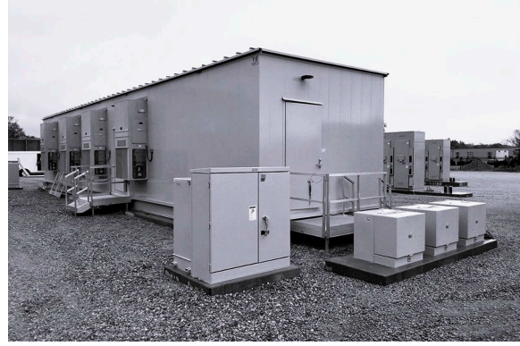
Power transformer. Source: CAT, 2017.
