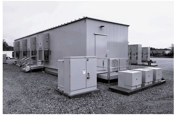
Power transformer. Source: CAT, 2017.
