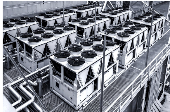
Rooftop air cooling system. Source: Area.
