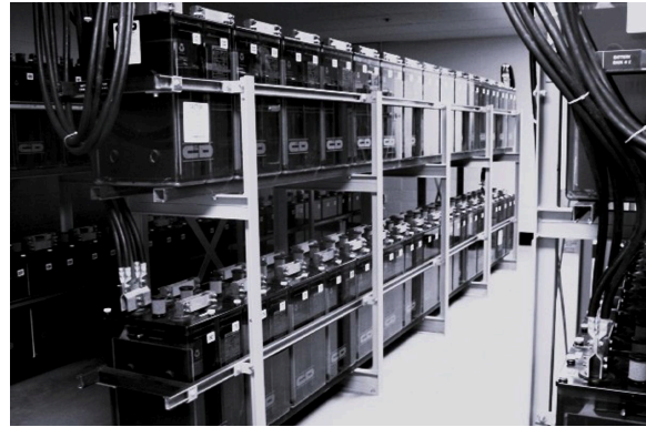
UPS batteries. Source: Kim Otte, 2010.
