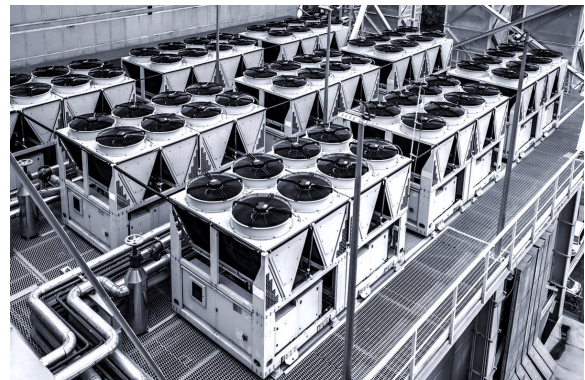
Rooftop air cooling system. Source: Area.
