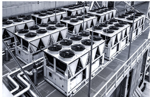
Rooftop air cooling system. Source: Area.
