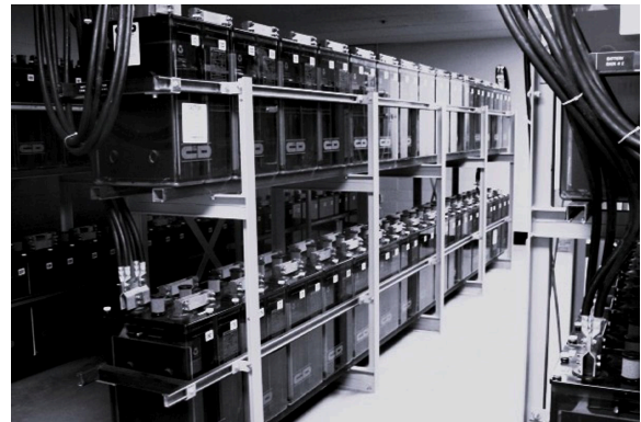
UPS batteries. Source: Kim Otte, 2010.
