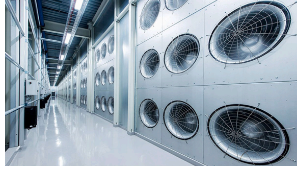
Interior cooling infrastructure of Meta's data centre in Luleå, Sweden. Source: Upsite Technologies, 2026.
