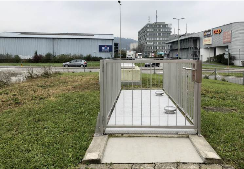
fig. 105 Drinking water from a depth of 35m Groundwater pumping well in the groundwater pumping station Ehrenhau, Regensdorf.
