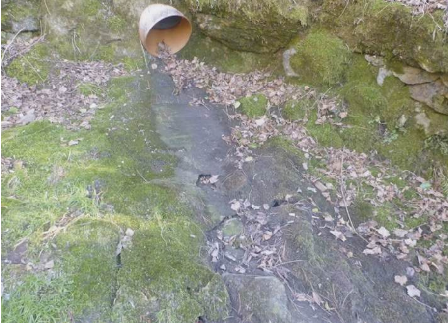
fig. 157 Water protection attempt Signage on an open residential shaft warning that a river branch is flowing underneath. Aim is to prevent the passer from throwing dirty water into the shaft.
