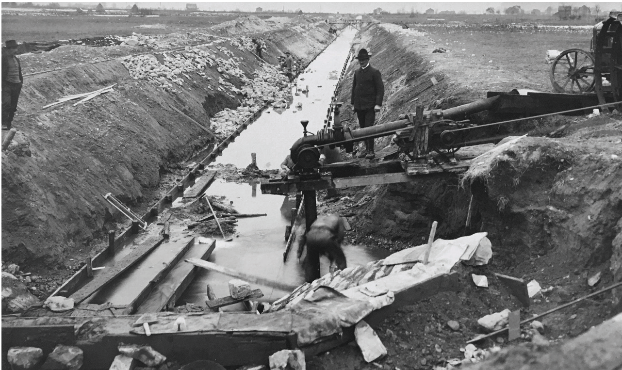
Construction of the Giessen, a new channel between Altdorf and Flüelen, as part of the melioration of the Reuss plain between 1919-1925. (Photo: PD)
