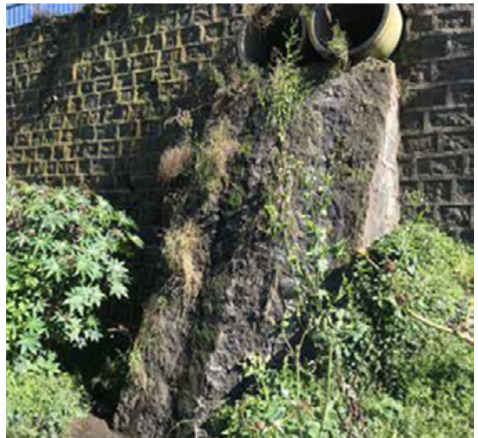
Sewage discharge into Kebena River
