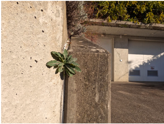
Flowering Growing Through Concrete Wall
