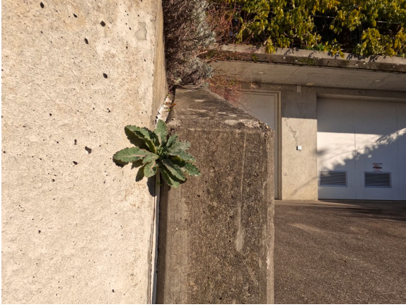
Flowering Growing Through Concrete Wall
