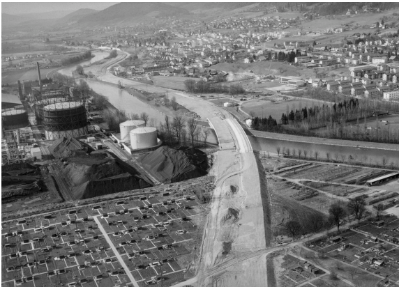
View on the construction of the highway A1 in Schlieren. Photograph: Comet Photo AG, 1969.
