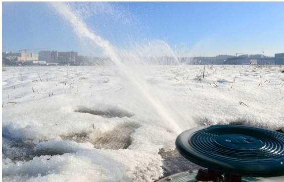
Sprinkler system to spray de-icing water over grassed areas. Source: Zurich Airport.
