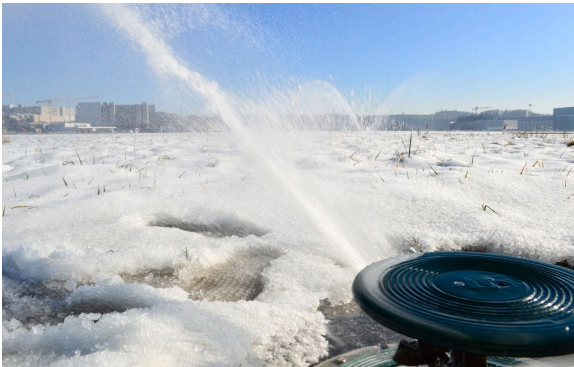
Sprinkler system to spray de-icing water over grassed areas. Source: Zurich Airport.
