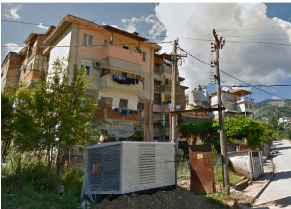
Electricity infrastructure in Gjirokastër, 2019. Photograph: Google Street View [ https://goo.gl/maps/BCi2T8Da9FTmZzWq9 ].
