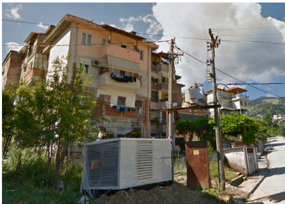
Electricity infrastructure in Gjirokastrë, 2019. Photograph: Google Street View [ https://goo.gl/maps/BCi2T8Da9FTmZzWq9 ].
