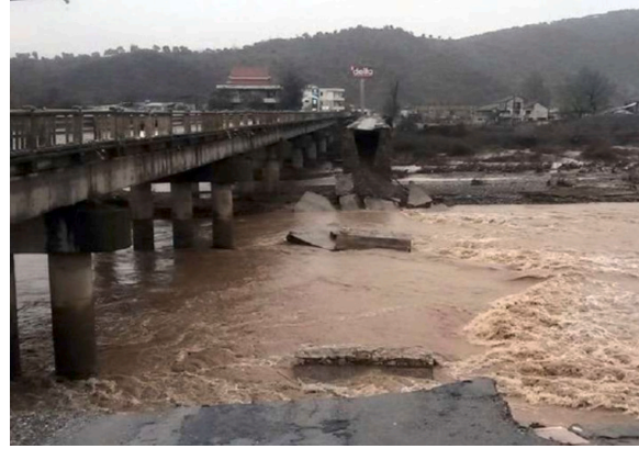
Collapsed bridge between in Dropull near Gjirokastër after heavy rainfalls in December 2017. Source: Periskopi [ https://www.periskopi.com/permytjet-neshqiperi-shemben-pese-ura-ne-gjirokaster/ ].
