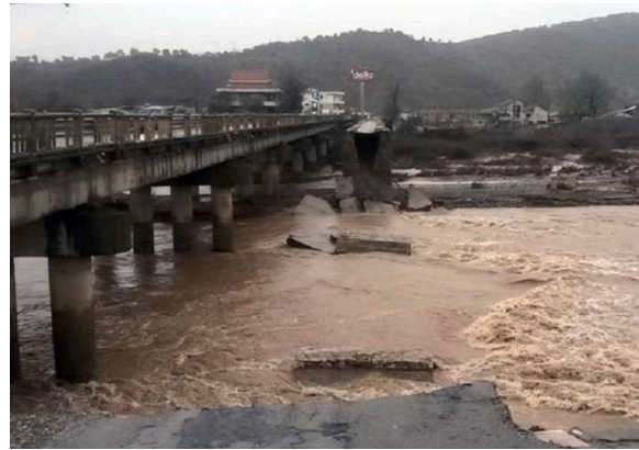
Collapsed bridge between in Dropull near Gjirokastër after heavy rainfalls in December 2017. Source: Periskopi [ https://www.periskopi.com/permytjet-neshqiperi-shemben-pese-ura-ne-gjirokaster/ ].
