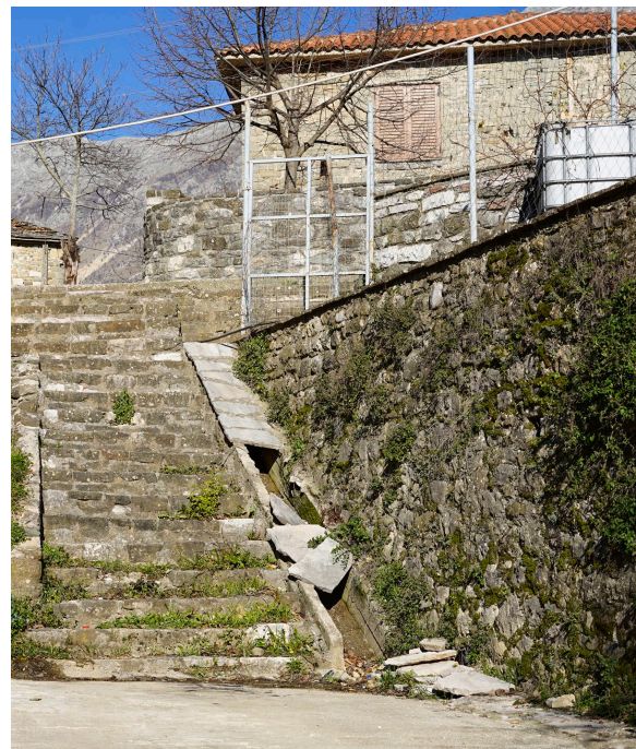
Dysfunctional water channel in Dhoksat. Photographer: Gylar Mydyti.
