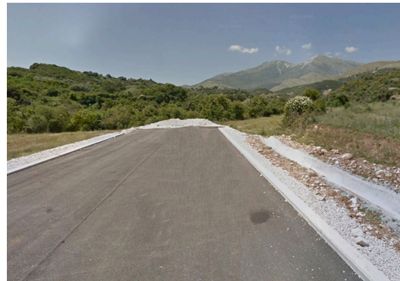
Construction of a new road between Kardhiq and Sarandë. Photograph: Google Street View [ https://goo.gl/maps/mynP4ka7tQzudoeW9 ].
