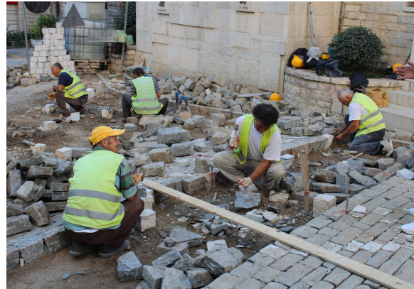
Workers refurbish a road in the city of Gjirokastër using traditional construction techniques. Photograph: Gylar Mydyti.
