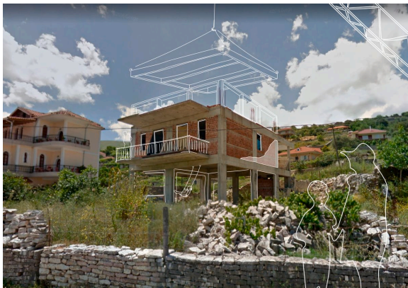
Perspective of the Jorgucat workshop in an unfinished house structure. Photograph: Gyler Mydyti, 2019.
