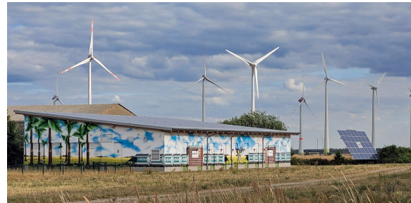
Battery station in front of wind turbines
