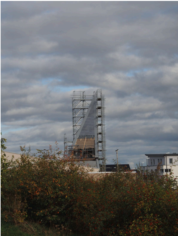
THE NEW CHURCH IN MORSCHENICH-NEU IS STILL UNDER CONSTRUCTION. Photograph: Dara Rüfenacht, 2022.
