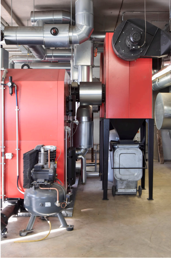
Stove of the central heating system in Morschenich-Neu
