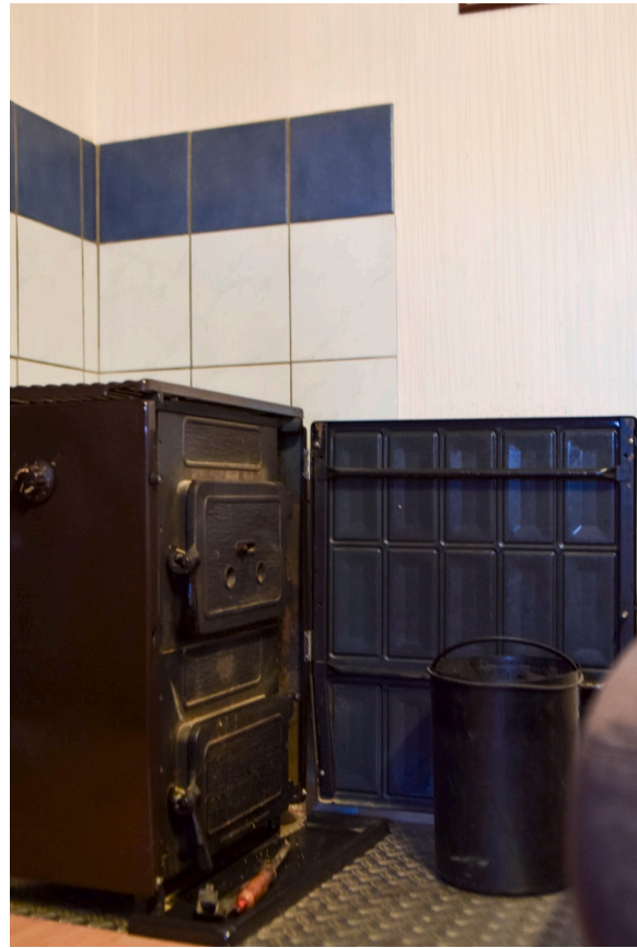
The coal stove in the living room.
