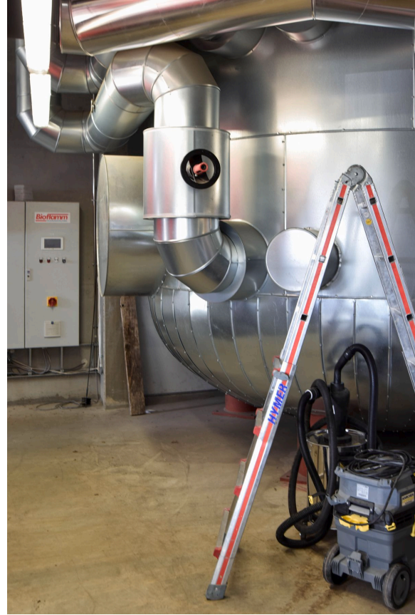
Heating storage unit
