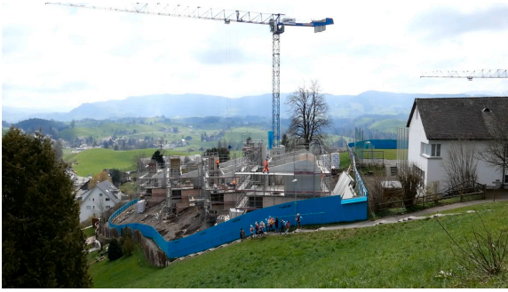
CONSTRUCTION SITE IN THE CENTRE OF THE VILLAGE. Photograph: By the authors.
