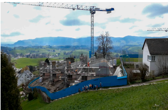
CONSTRUCTION SITE IN THE CENTRE OF THE VILLAGE. 5 APRIL 2023. Photograph: By the authors.
