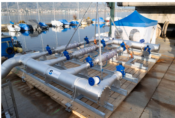
Pipes In the Lake. Source: powernewz.ch, 2022. [ https://www.powernewz.ch/rubriken/waerme-und-kaelteversorgung/seewasserverbund-bahnhofstrasse/ ]
