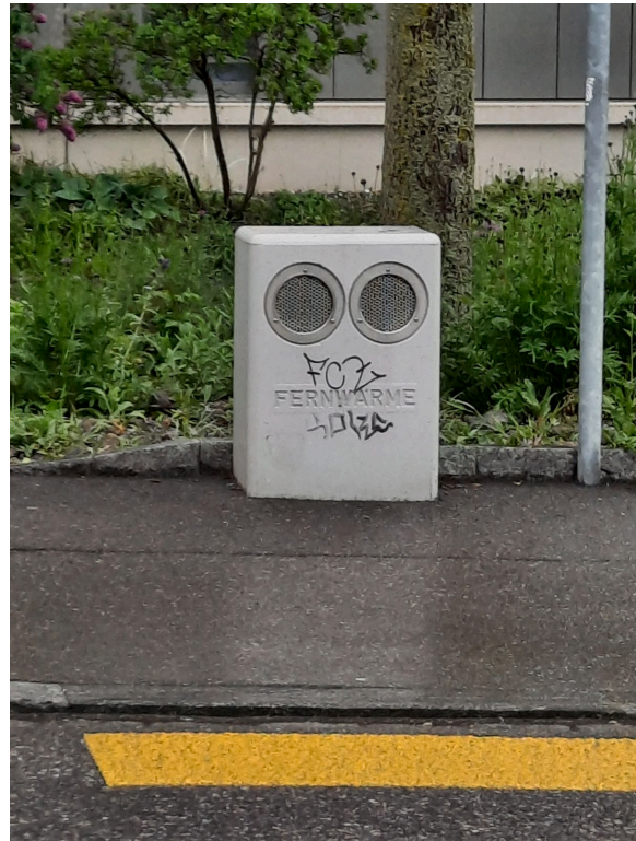
Ventilation Box at Neunbrunnenstrasse, Oerlikon. Source: Own Picture, 2024.
