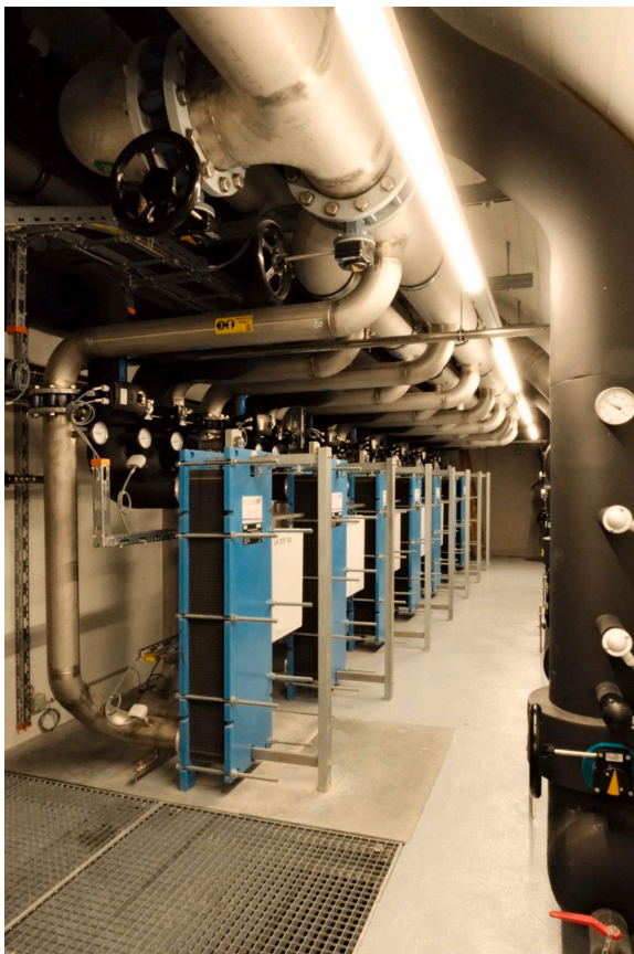
Water-to-water heat exchanger. Photograph: the authors, 2025.
