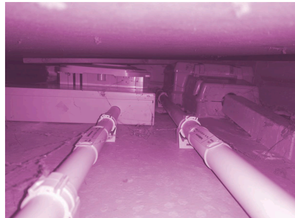
OPTIC FIBRE SERVICE ENTRANCE
