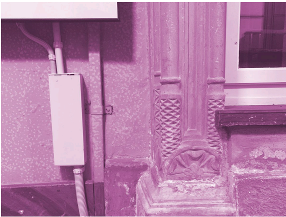
OPTIC FIBRE SERVICE ENTRANCE
