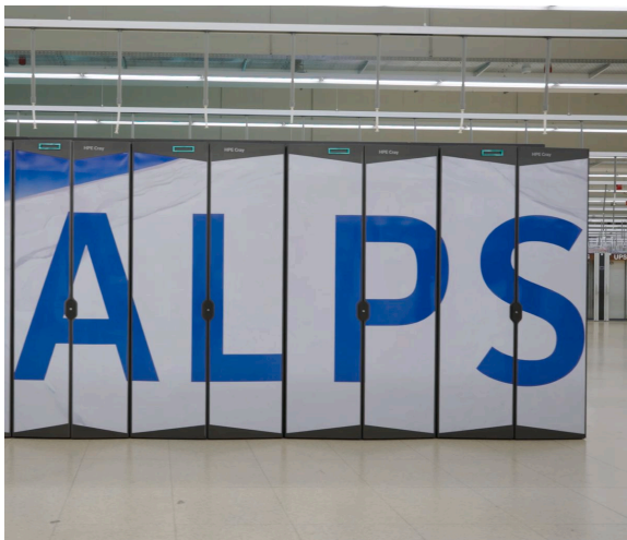
ALPS supercomputer. Source: CSCS, 2024.
