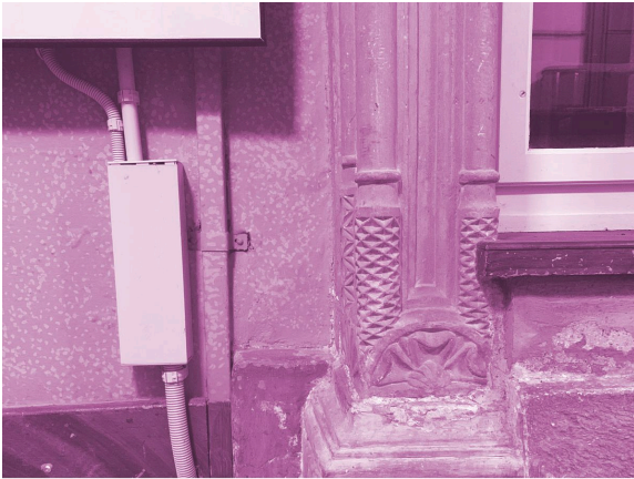
OPTIC FIBRE SERVICE ENTRANCE
