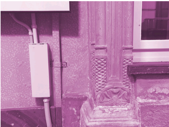
OPTIC FIBRE SERVICE ENTRANCE
