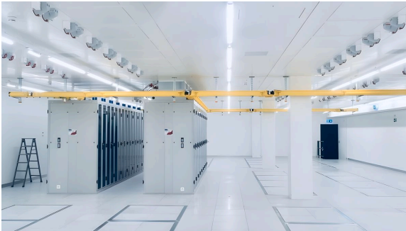
Inside Swisscoms data centre Herdern (AI-enhanced by authors), approx. 2020: Source: MBA Projektmanagement.
