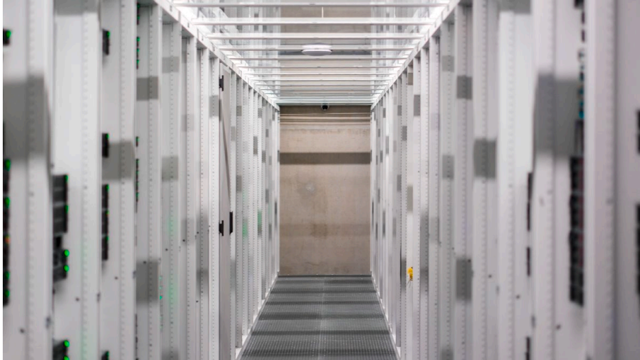
INFOMANIAK DATA CENTRE, GENEVA. Photograph: film still from Close Encounters: Bits with Benefits? , the authors, 2025.
